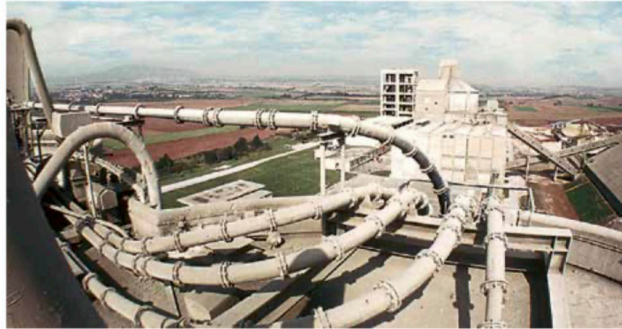
Pipes used in the cement industry are reliably protected with ABRESIST, KALCRET or – in case of extreme wear – with KALCOR and KALOCER
