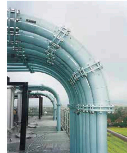
Protection for pneumatic and hydraulic pipes
