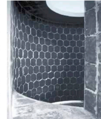
Extended service life of plant components
