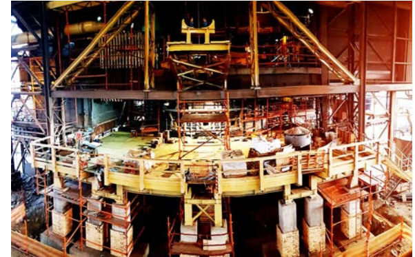
FURNACE MECHANICAL PROJECTS
